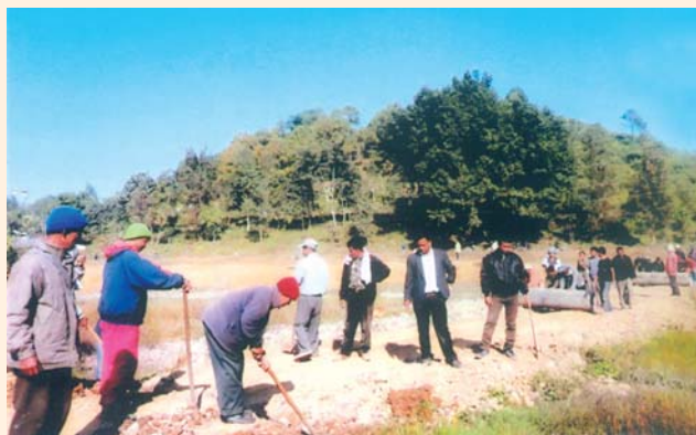
MGNREGA job card holders levelling the road and laying of culvert at Sagang Village in Churachandpur District (Manipur)
